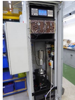
Gaseous Activity Monitoring (GAM) system at Hartlepool power station
