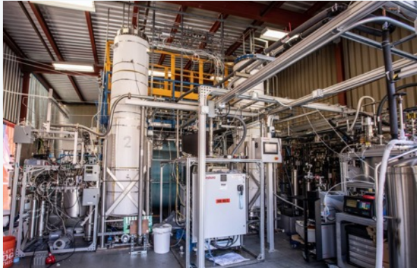
Krypton removal system at SLAC
