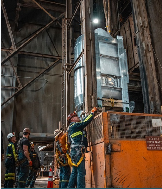
ICV transport underground
