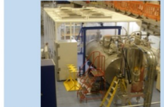
Figure 3. A picture diagram of the large cryogenic system used in CREF, and its connection to the CREF cleanroom.
